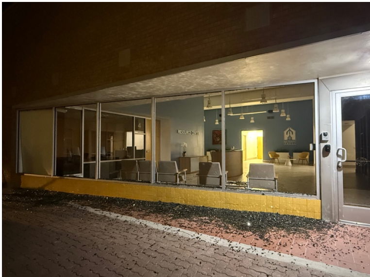
Damages the date of the incident - August 5, 2025
