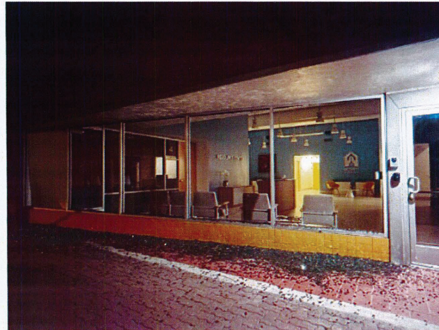
DAMAGES TO FAÇADE
