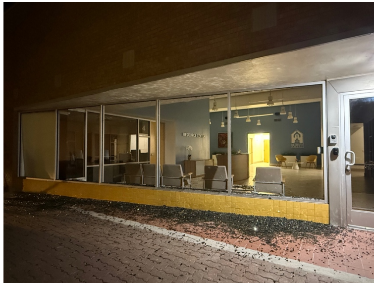
Damages the date of the incident - August 5, 2025
