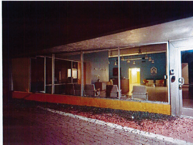
DAMAGES TO FAÇADE
