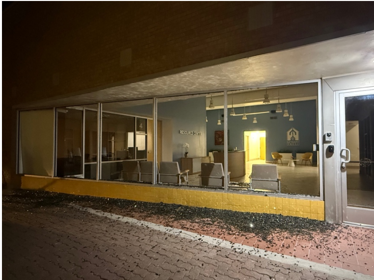
Damages the date of the incident - August 5, 2025
