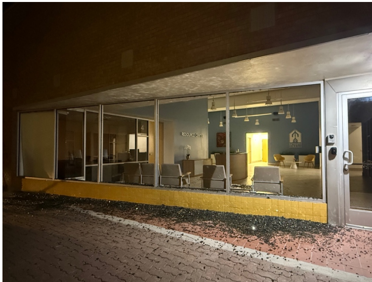
Damages the date of the incident - August 5, 2025
