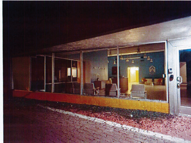
DAMAGES TO FAÇADE
