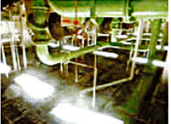
LC South Campus New Chiller
