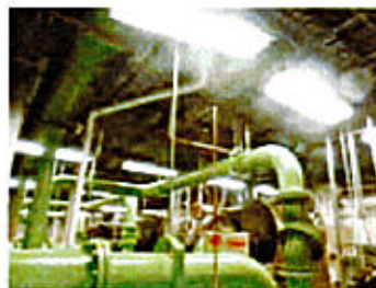
LC South Campus New Chiller
